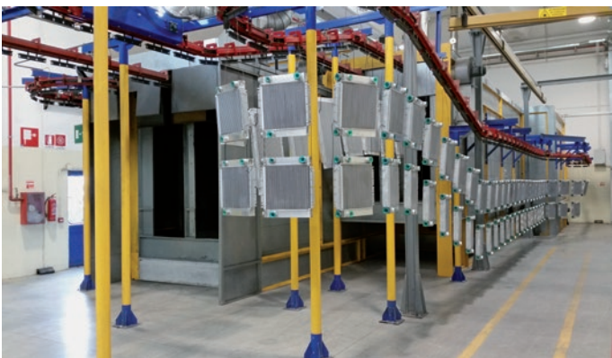
Paint shop (powder coating)
